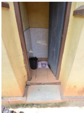
Figure 6 Make enough space and brightness
